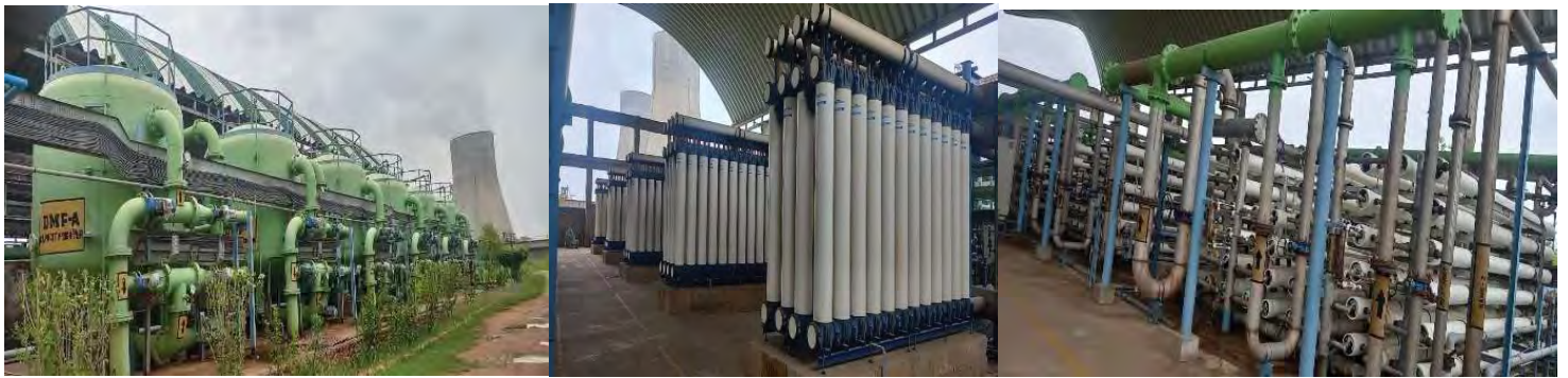
Effluent Treatment Plant
